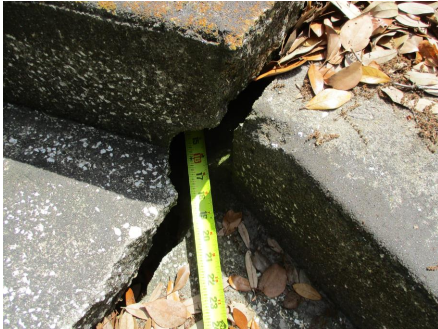
Void under Settled Section of Wall
