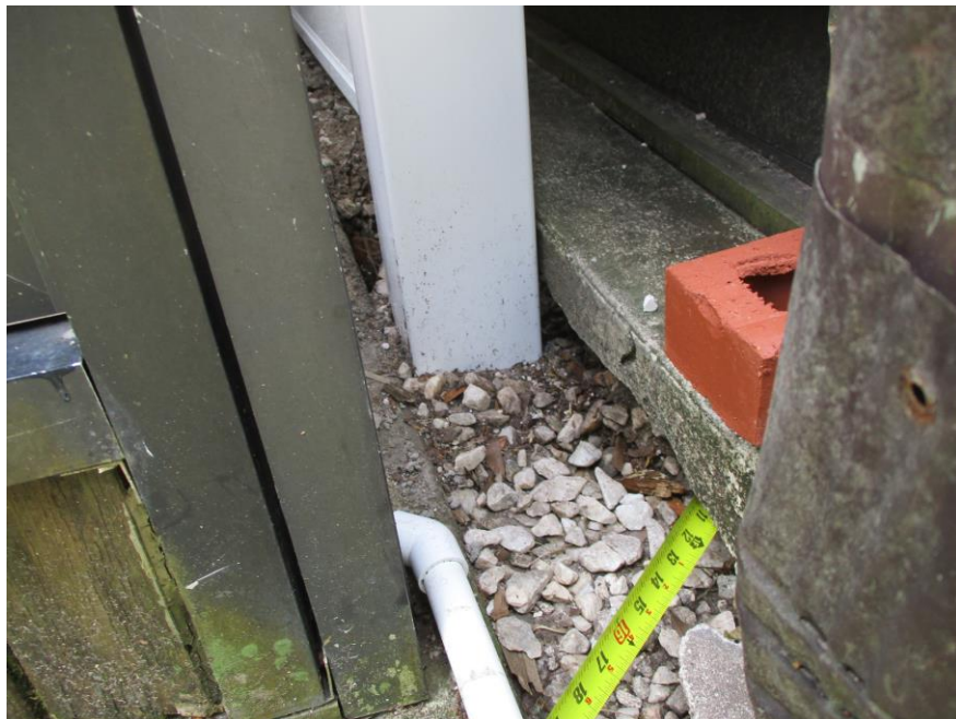
Void under Existing Patio Slab
