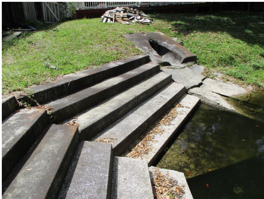
Settled Wall Section at West End
