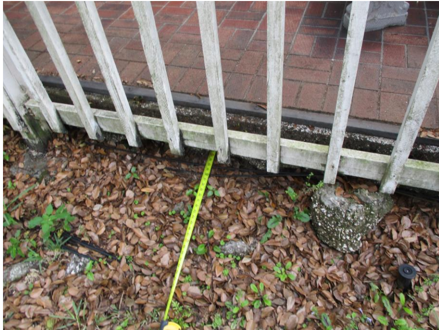
Void under Existing Patio Slab
