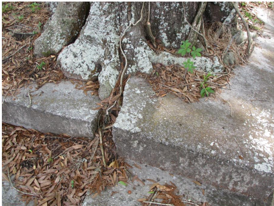
Tree Growing next to Seawall causing Damage
