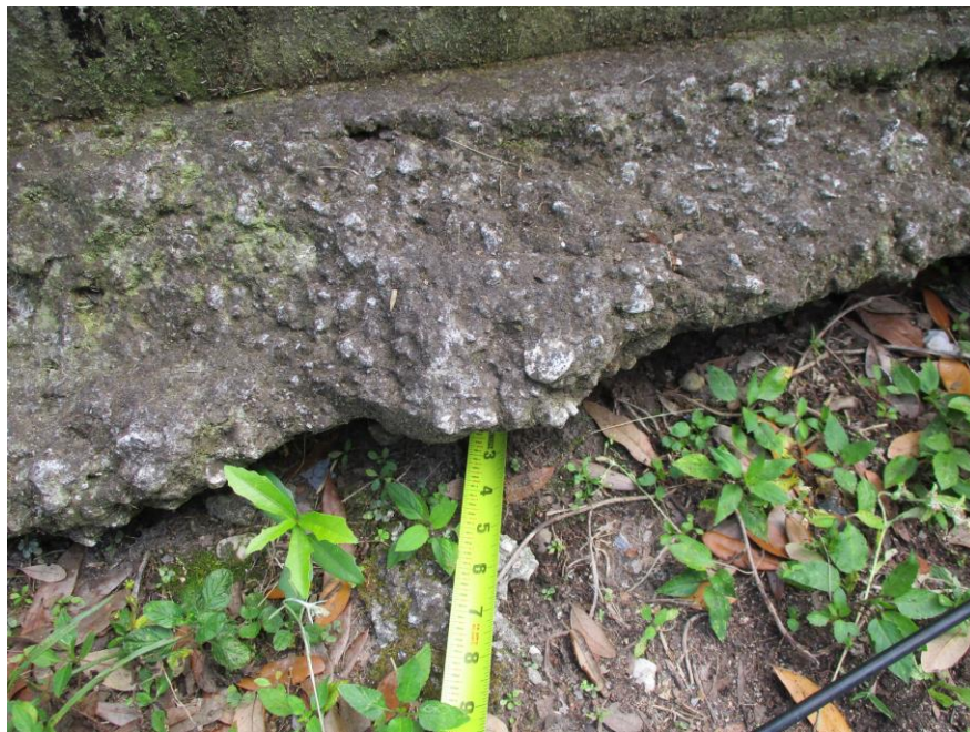
Voids under Existing Fence Footing
